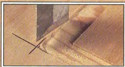
Use a chisel, with its bevel facing the recess, to remove excess corner material in a line parallel to the recess.
