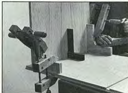
Clamp the bottom, shelves, and top into the dados, using scrap braces to keep them square until the glue dries.
