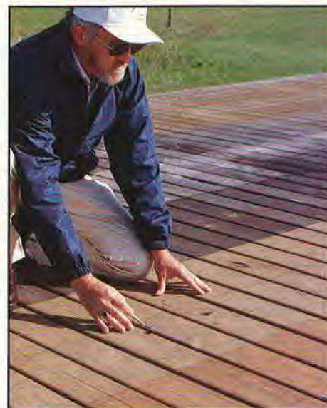
At the Valley View exterior finish testing facility, Bill Feist inspects the wood on a test deck for finish durability.
