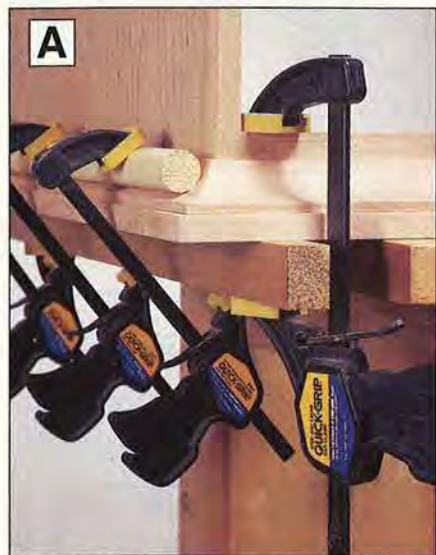
Use a dowel and clamp block when clamping the cove molding to the top of the cabinet.
