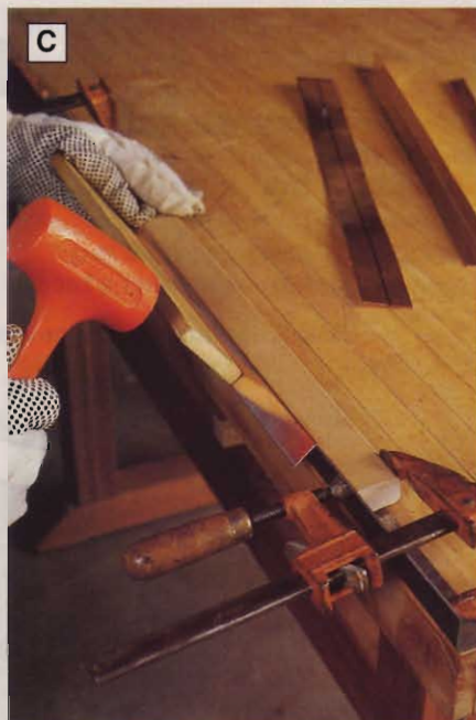
For straight, even bends, use a long block of wood when forming the copper ridge caps.
