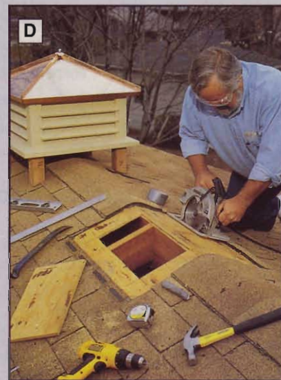
Mark the cutlines, remove all the nails, and use a circular saw to cut the opening to size.
