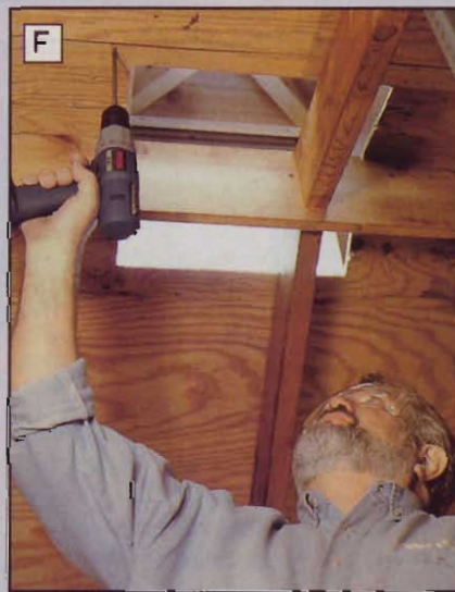
F Using a helper on the roof to hold the cupola in place, drive screws through the roof sheathing into the cupola corner posts.
