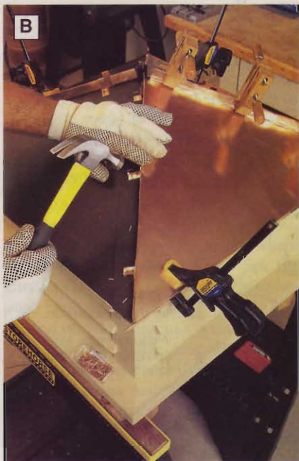
Use the copper clips to secure the copper roof panels to the roof sheathing.
