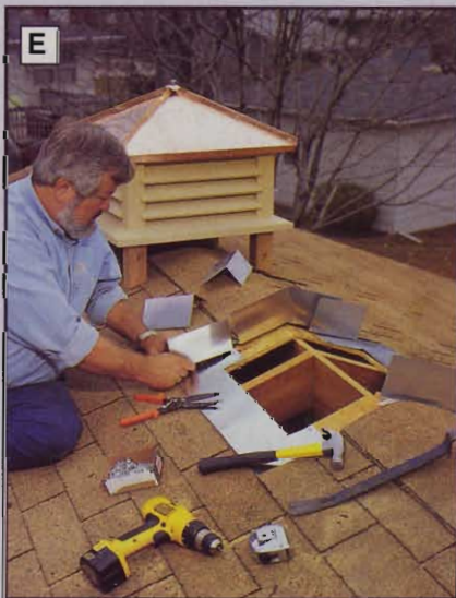
E Bend pieces of flashing, and slide them under the shingles along both edges of the opening.
