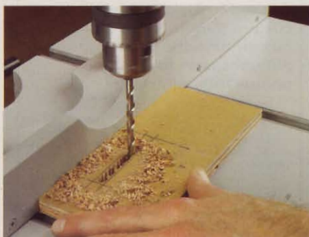
6 DRILL OUT THE WASTE Using a bit \frac{1}{8} " smaller than the slot width, drill overlapping holes inside the layout lines. Note: Creating a slightly undersized rough slot with a drill bit lets you rout a clean finished size slot in one easy pass.
