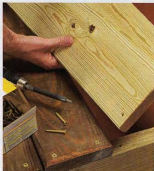
Use "The Yankee Flip" as a thrifty way to revive the look of weathered deck boards.
