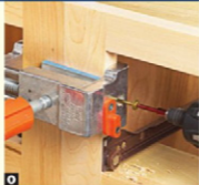
O To join cabinets, flip down the drilling guide and drive a panhead screw into both frames. Use at least two screws to connect frames.
