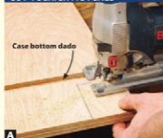
A A toe kick allows you to stand closer to a cabinet without bumping the front with your feet. Cut these clear of the case bottom dado.
