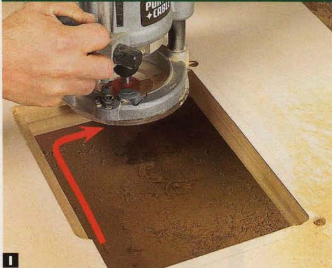
I Rabbet clockwise between the drilled holes with a bearing-guided bit to create a lip that will accept the insert.
