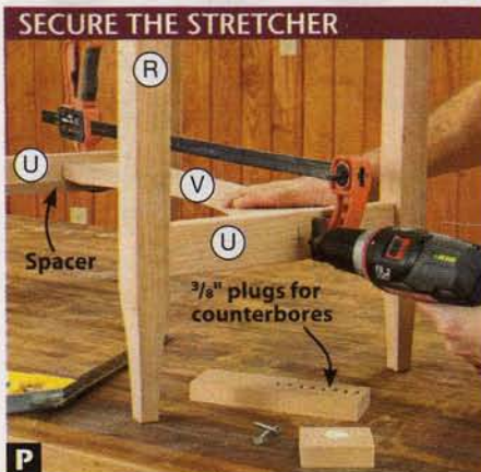
P Temporary spacers hold the stretcher (V) while drilling counterbores and screw holes. Plug the counterbores after driving screws.
