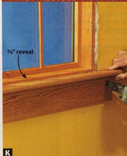
K Align the stool/apron assembly with the sill edge reveal marks, and attach the assembly to the wall with 15- or 16-gauge nails.
