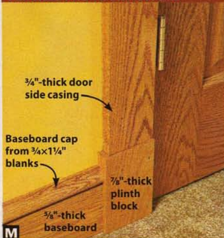
M A plinth block at the base of the door jamb provides a transition between the side casing and baseboards.
