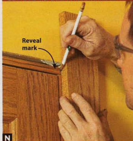
N Transfer the reveal mark on the door head jamb edge to the edge of a door casing. Then trim the casing to that mark.
