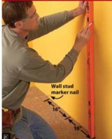
From a nail marking one stud, mark the remaining studs every 16". Use a level to transfer marks for nailing the chair rails.
