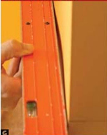
A wall dip this severe needs to be patched with joint compound, primed and repainted before you install a chair rail.
