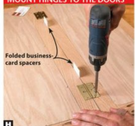
H Center and screw on the hinges between two doors separated by a folded business card that acts as a spacer.
