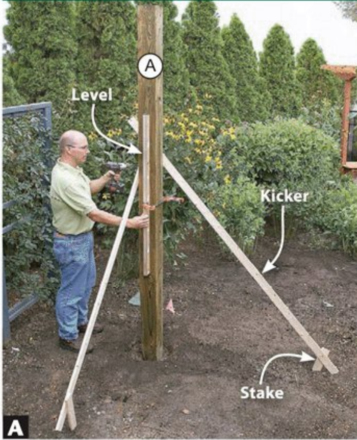
A Brace the post (A) with kickers and stakes. Check for plumb in both directions before and after adding concrete to the hole.
