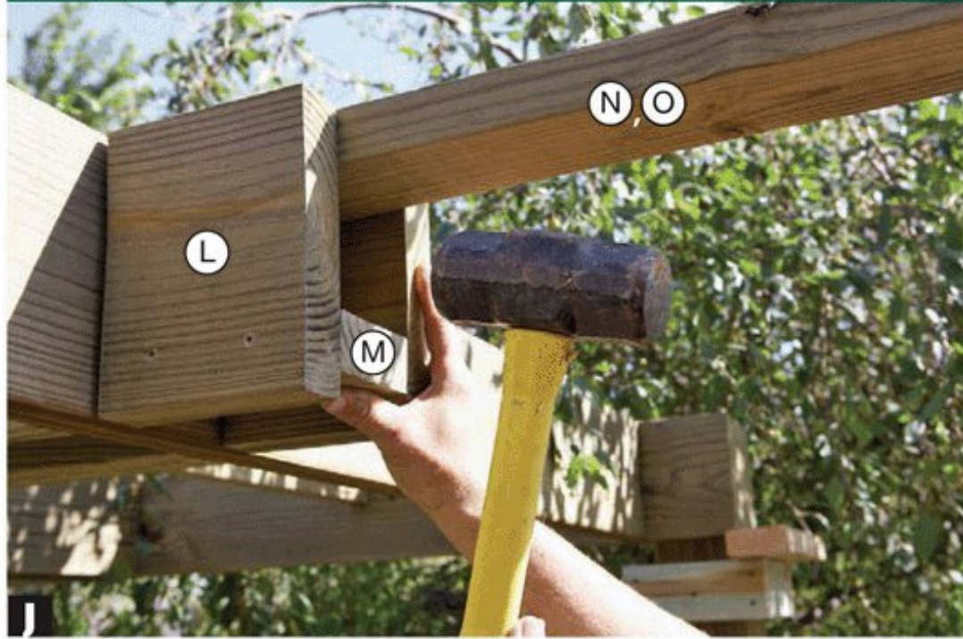
J Straddle the cross ties (N, O) with a beam filler (L/M). Strike the filler sides to mark the locations of the lag-screw heads.
