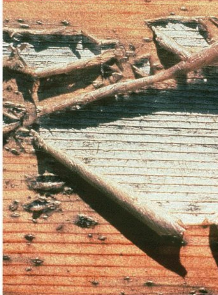
Clear film finishes adhere only to the top layer of cells. When the wood sheds the sun-damaged cells, the film quickly sloughs off.
