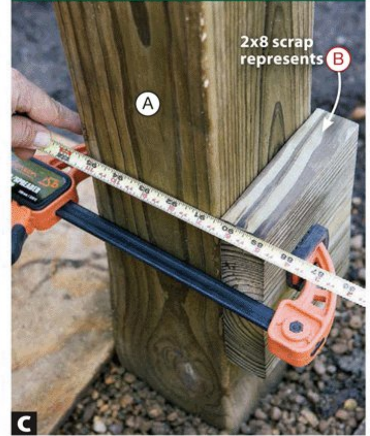
C Clamp a 2×8 scrap to each post to represent the inside beams (B) when measuring for the length of the crossbeams (C).
