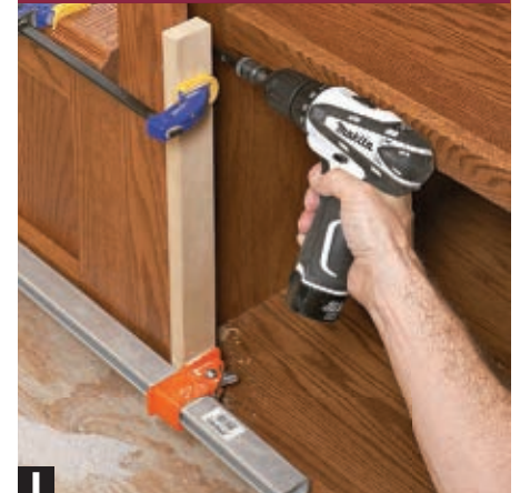
I Pull the bookshelf cabinet and window seat tightly together using clamps before drilling pilot holes. Doors will help hide the screws.
