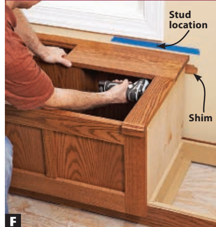
F Marked painter's tape shows stud locations where you'll drive mounting screws through the window-seat back and into the wall.
