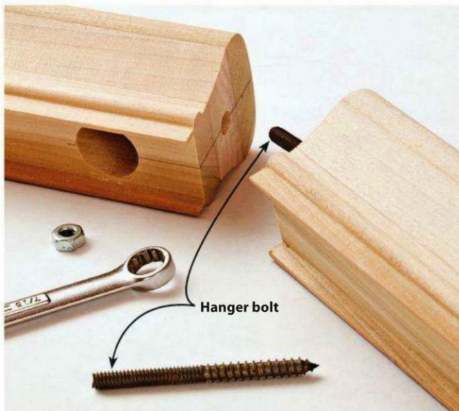
An end-to-end handrail joint works much like a bed-frame joint. The nut on the hanger bolt pulls the butt joint tight.
